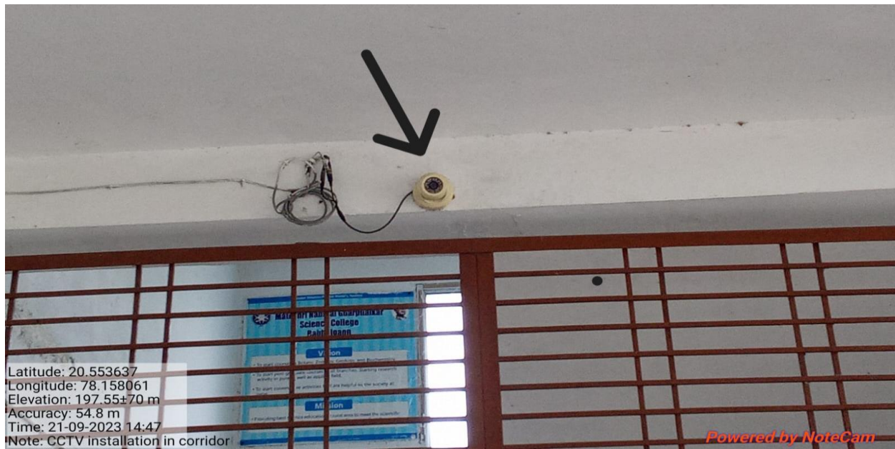
CCTV CAMERA INSTALLATION IN CORRIDOR
